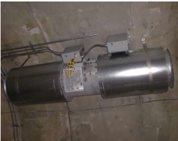
Jet fan installed in the Washington Dulles Airport.
