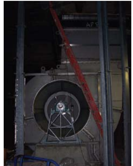
This is one of the twenty-three 316L stainless steel centrifugal fans installed in the Queens Mid-Town Tunnel in New York.
